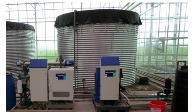
Figure 12. Standard dosing unit for drip irrigation (right) and UV disinfection unit (left).
